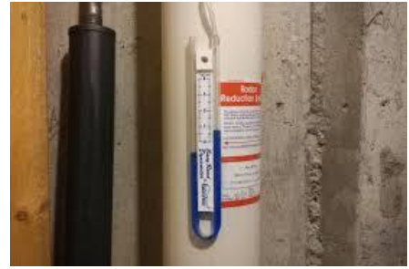
Figure 4.3.6.5-: Radon System Manometer in Basement (Scott Home Inspection, 2017) (Radon, 2024)
