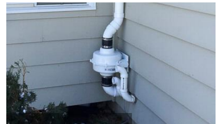
Figure 4.3.6.5-2: Radon Mitigation Systems (Scott Home Inspection, 2017) (Radon, 2024)
